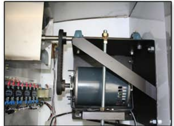
New indirect fan system keeps the motor cooler and eliminates motor failure due to out of balance, dirty fan blades.
